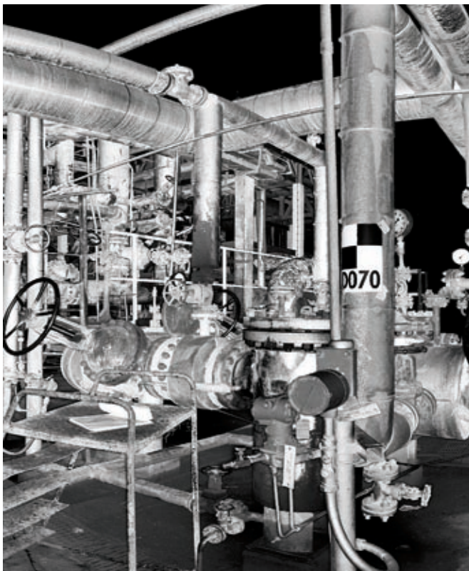
FIG. 2 Actual laser documentation (not a picture) for refinery equipment. Each point is a highly precise measurement.
