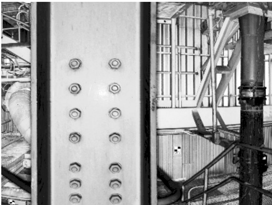
5. The nuts and bolts of laser scanning. Note the fine level of detail, including bolt threads, in this laser scan image of a power plant’s structure and components. Courtesy: Quantapoint Inc.
