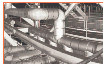
Quantapoint 2D As-Built Laser Documentation for a Power Plant (not a picture)
