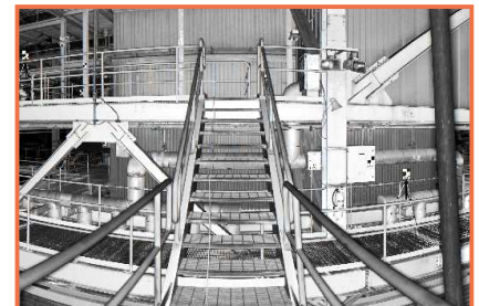
Quantapoint 2D As-Built Laser Documentation for a Power Plant (not a picture)
