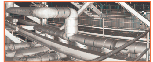
2D Image of Quantapoint Laser Scan for a Power Plant ( not a picture)
