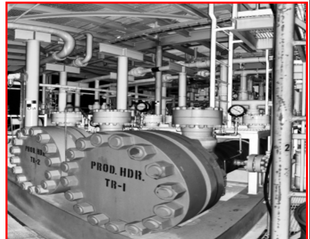
Quantapoint 2D Laser Scan (Not a Picture) Each Point is a Measurement
